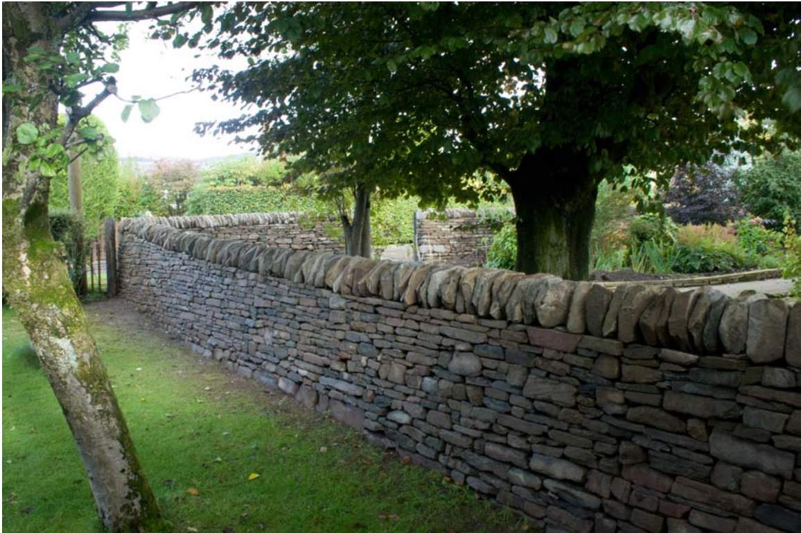
Boundary wall at 10 Kellyburn Park, Best Small Project, Dollar Civic Trust Awards 2008 The judges were impressed with the workmanship and quality of finish on the wall. (Denfind Stone) Photo: J. Hoffman
