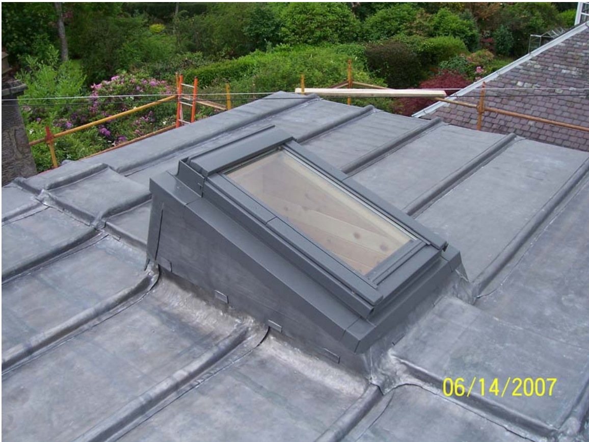
Roof Restoration at 26 Harviestoun Road, Highly Commended Restoration/Conservation Project The research and attention to detail are outstanding and ensure that local architectural heritage is conserved and enhanced for many years to come (painstaking attention to detail) Photo: D. Brimer
